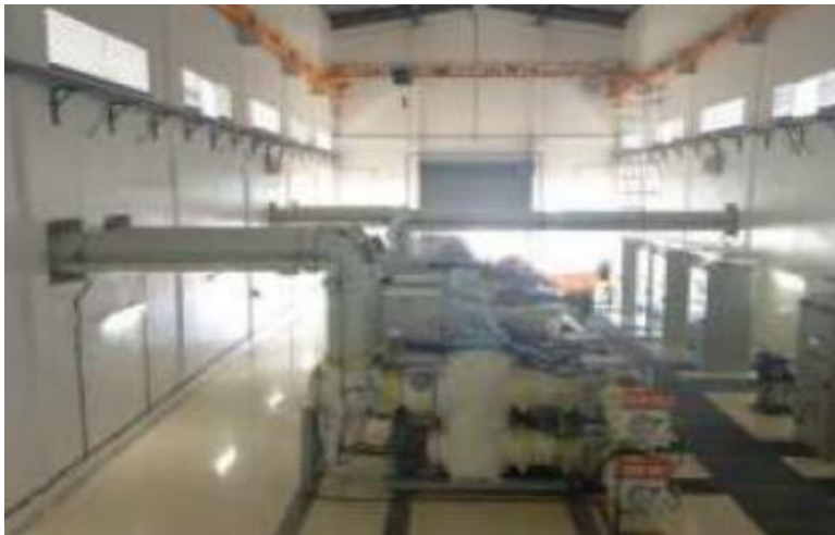
EGAT Substation 100% completed
